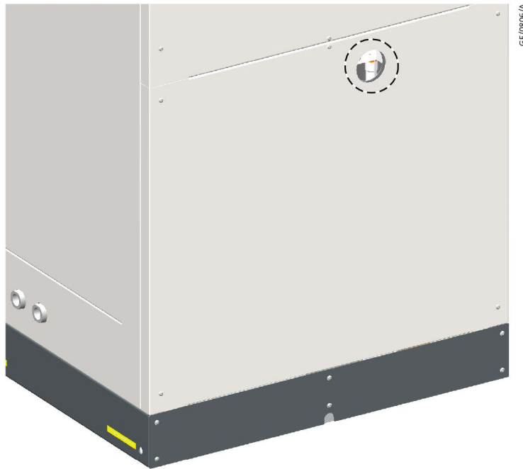
Figure 83 Pressure gauge on back of refrigeration unit
